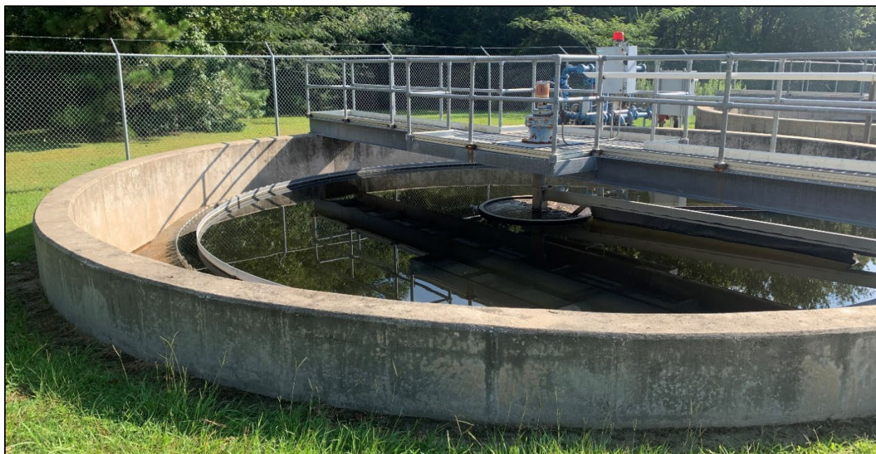
A WASTEWATER TREATMENT PLANT
